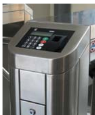
Integration with Access Control
